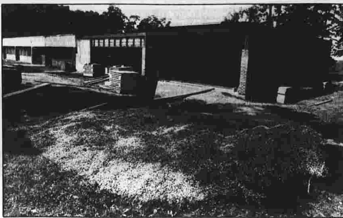
MORE SPACE — A two-classroom addition is currently being built at Bolton Elementary School to handle increased enrollment. Educators think more space will be needed in the next decade.
